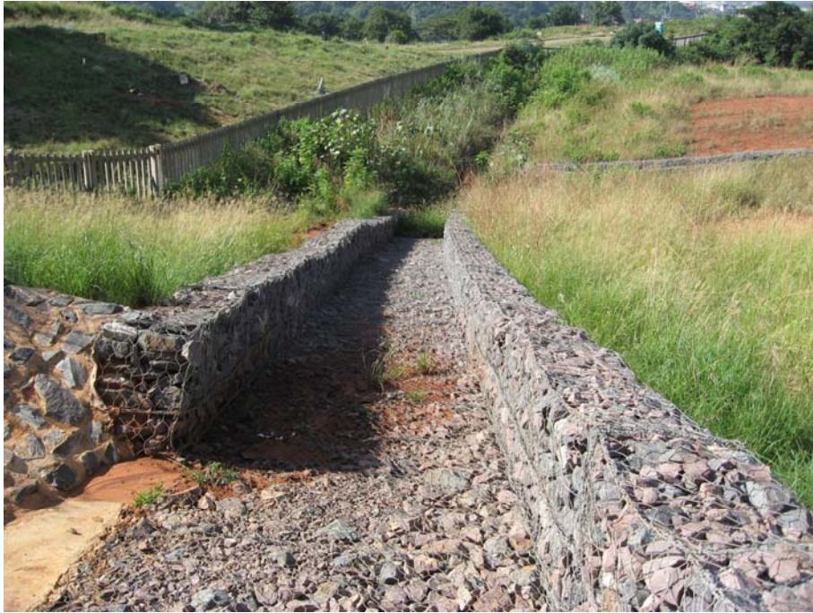
Plate 3: One of the newly completed drainage channels from the top of the site.
