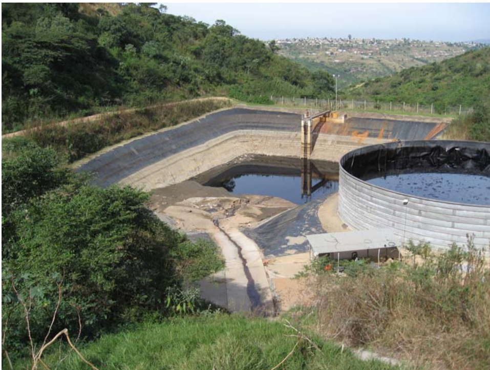
Plate 4: View of the Contaminated Storm Water Dam and the Leachate Storage Tank: note the silt in the dam.
