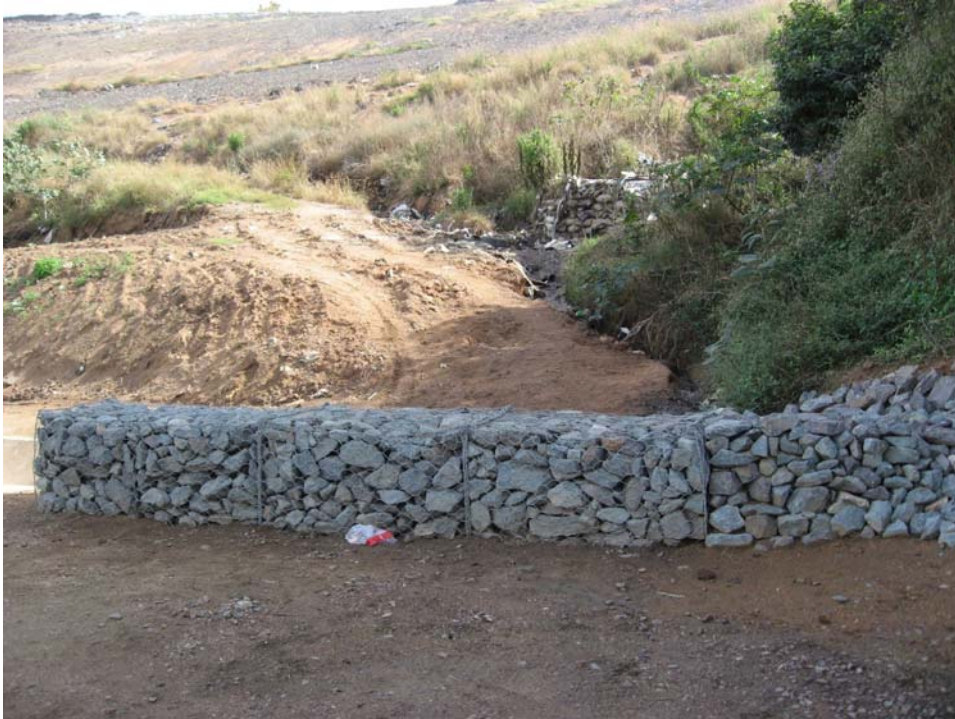
Plate 5: Barrier that has been place near toe of site in another attempt to minimise damage due to heavy rain
